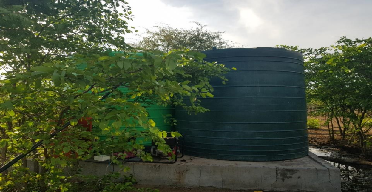
Illegal Connections to BH 9642 within Ranch NN-91. The dominant Mophane trees are going to be cleared
